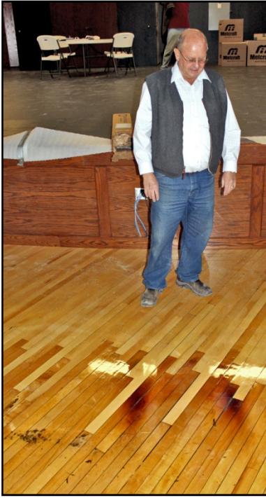
Dave Taylor inspects floor: City planner Dave Taylor examines burn marks where a stove once warmed the dance hall. The floor is the only remaining element of the Eclipse Pavilion constructed in 1895.
